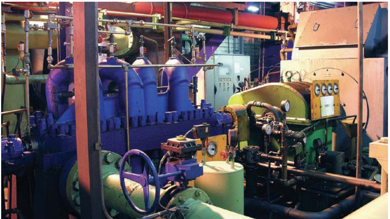
Significant energy savings can be gained by using VFDs to lower speed or flow by just 20 percent.
