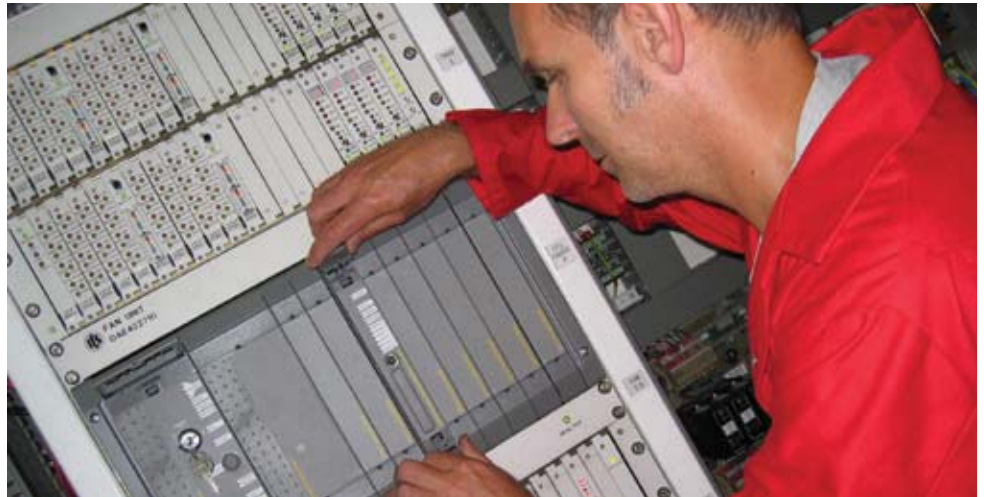
ICS Triplex's flagship solution is the SIL 3-rated "Trusted" fault-tolerant safety controller.
