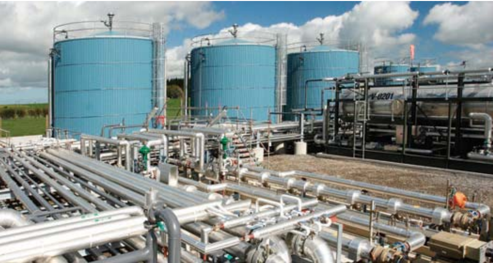
A network of pipes and pumps at the Cheal oil field in New Zealand extracts oil from nearly a mile beneath the surface and carries it through the production process.
